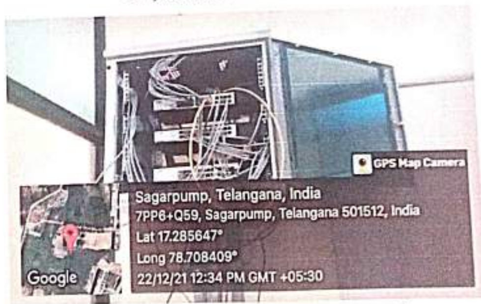
Internet Connection, Ground Floor
